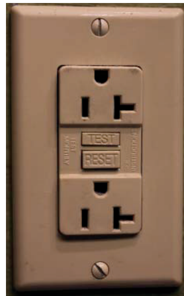
Make sure Ground Fault Circuit Interrupters (GFCI) are used in the shop area on the farm.
